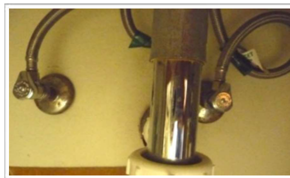
Accessible shut off valves
